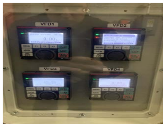
A VFD issue at Whippoorwill Pump Station.
