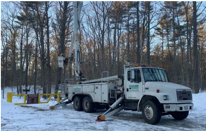
Damaged tree at the Blue Management Road gate is cut down.
